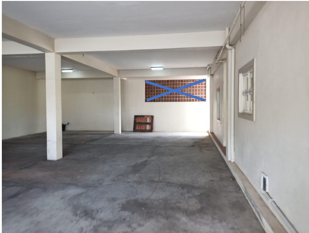
Figure 5. Eastern end of carport showing wall with fancy blocks to be demolished
